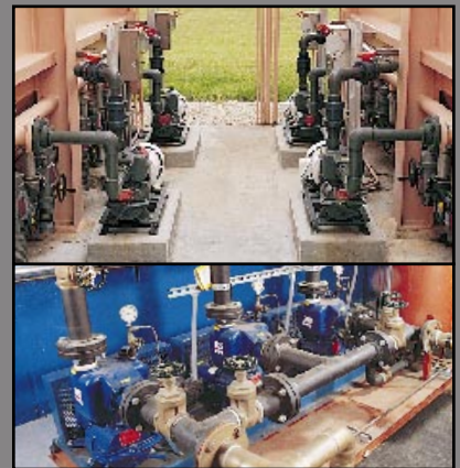
10 Series® pumps are used to transfer 110° wastewater from washing machines to the filtration system and heat exchanger at a commercial laundromat in Ohio, USA.
