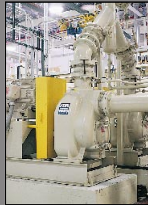
T Series™ pumps transfer coolant from the sump to filter and back to CNC machines at an automotive manufacturing plant in Michigan, USA.
