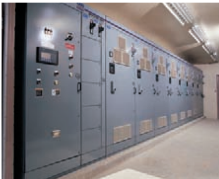
The Gorman-Rupp team of electrical engineers can design and supply a variety of control configurations to meet your needs.
