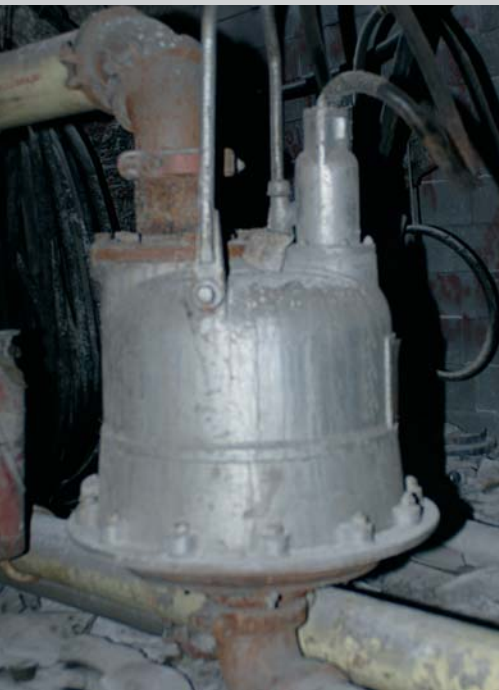
In-line staged submersible pump in a coal mine.
